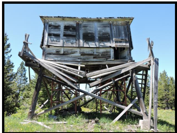
Barren Peak Lookout in 2016 before it Collapsed
